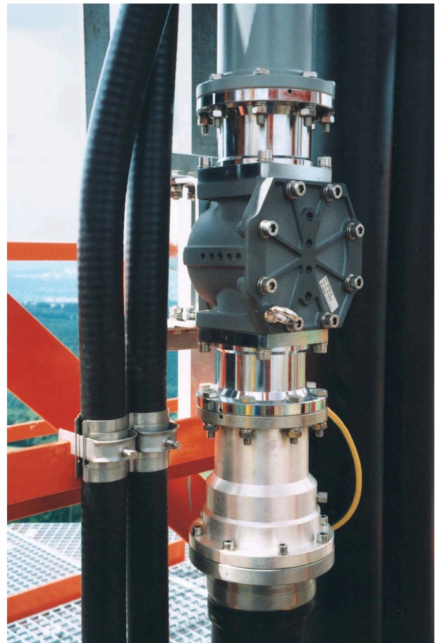
Measuring link in a cable run
